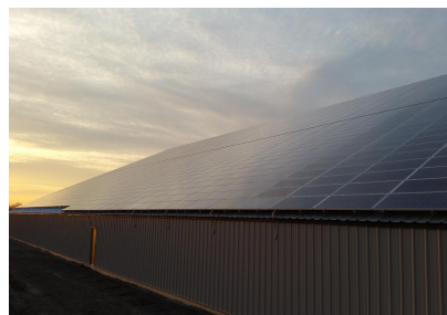
HCE's Solar PV installation at a Warehouse facility in Port Dover, ON
